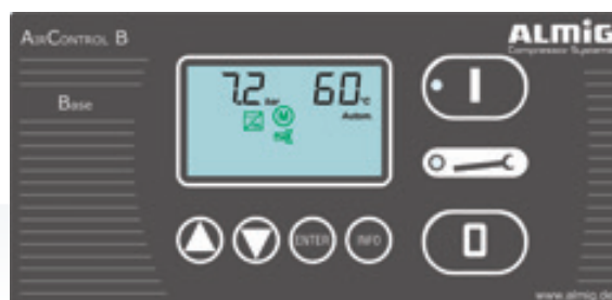
Air Control B
